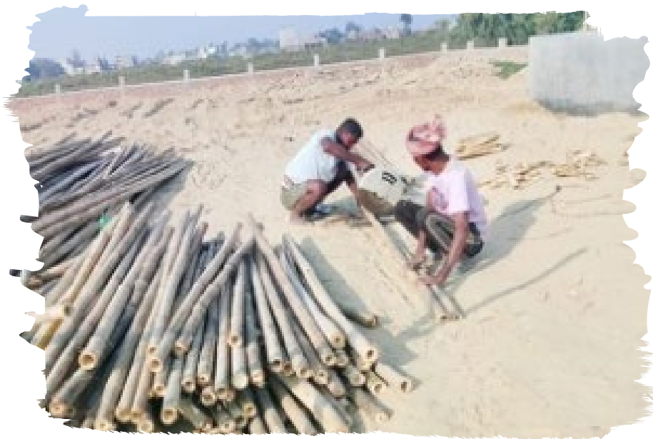
Community Improvement Center's bamboo treatment plant.
